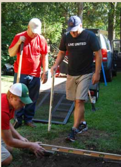
Employees from Roper St. Francis created a stable and level foundation before installing a new set of stairs for Albertha Robinson.
